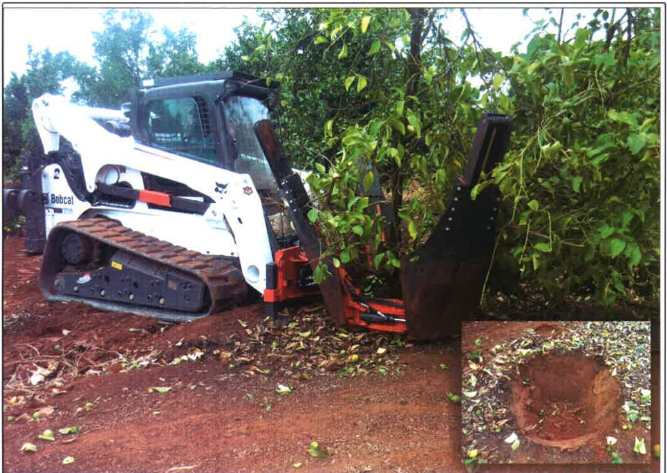
Bobcat T870B compact loader digs up, transplants and packages trees for Ihlathi.
